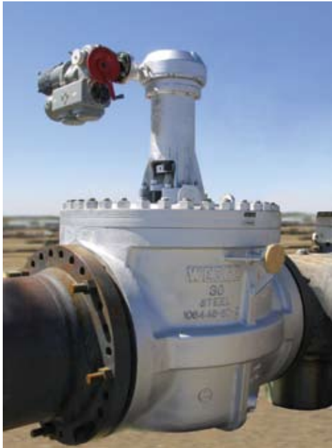
Wedgeplug installation at Suncor Millennium 2 Coker project, Fort McMurray, Alberta Canada. Electrically actuated 30" full port Wedgeplug, overhead vapor line isolation service.
