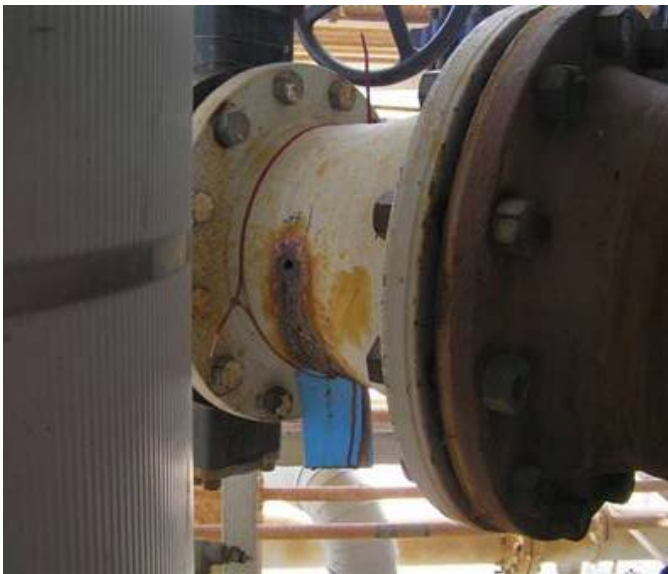
Appearance of a Leak
