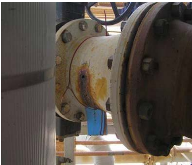
Appearance of a Leak
