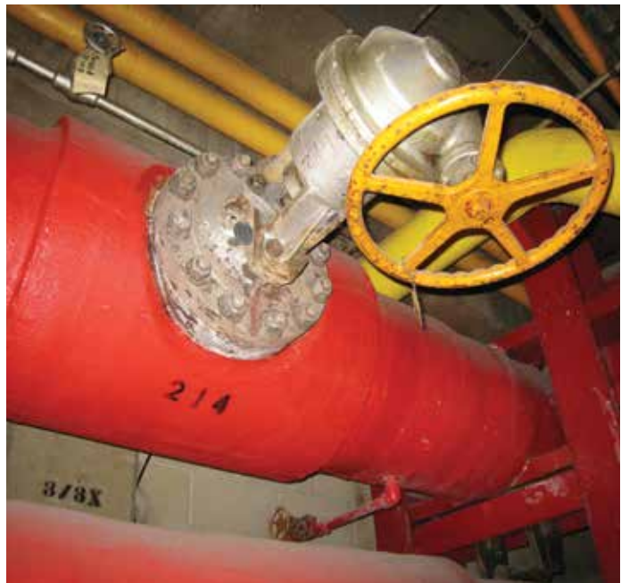
Wedgeplug installation at Chicago's O'Hare Airport. O-ring style plug used to supply water to the airport and also used in hot water loop to melt ice on runways.
